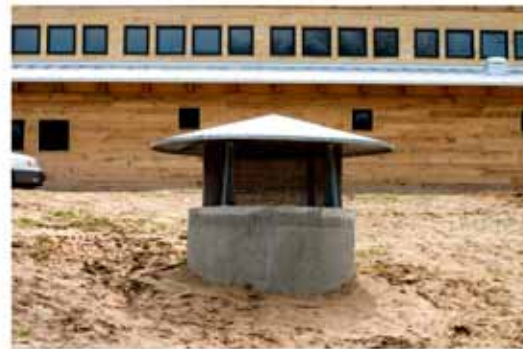
Outdoor air intake for main building
