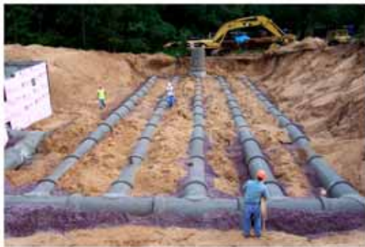
Earth tubes for air pretreatment
